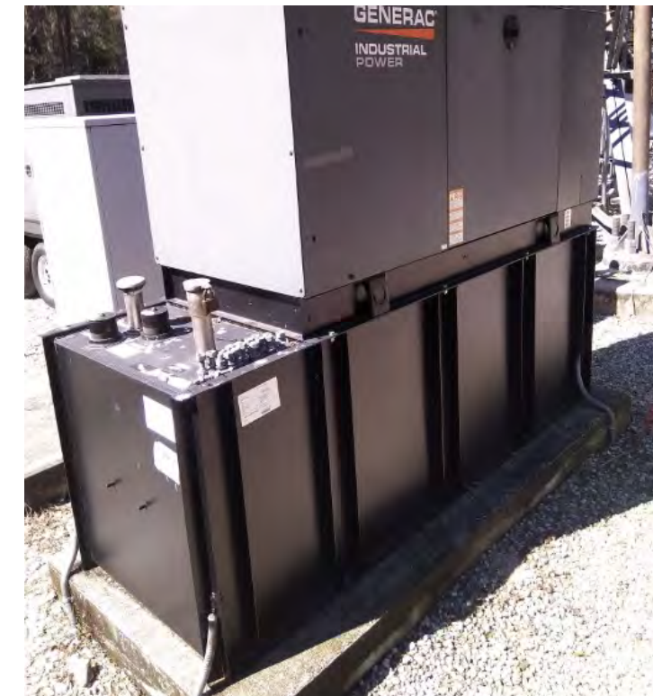
View of second emergency generator tank on-site.
