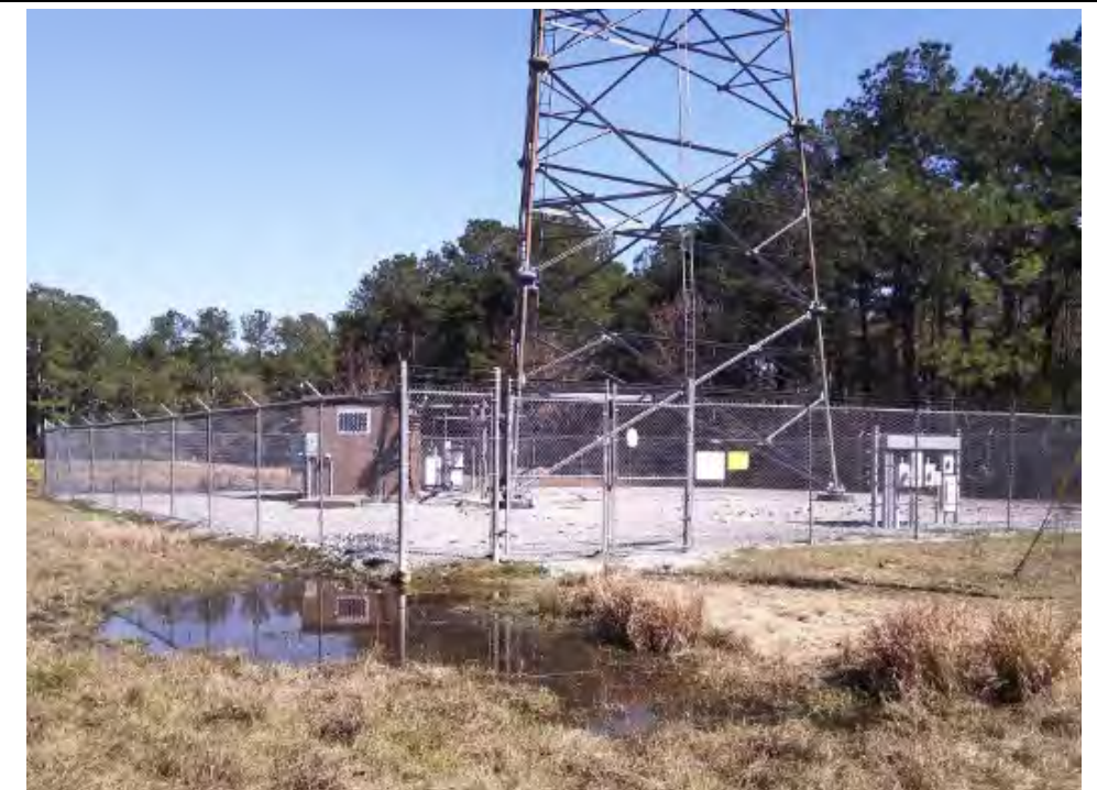
View of the radio tower enclosure.
