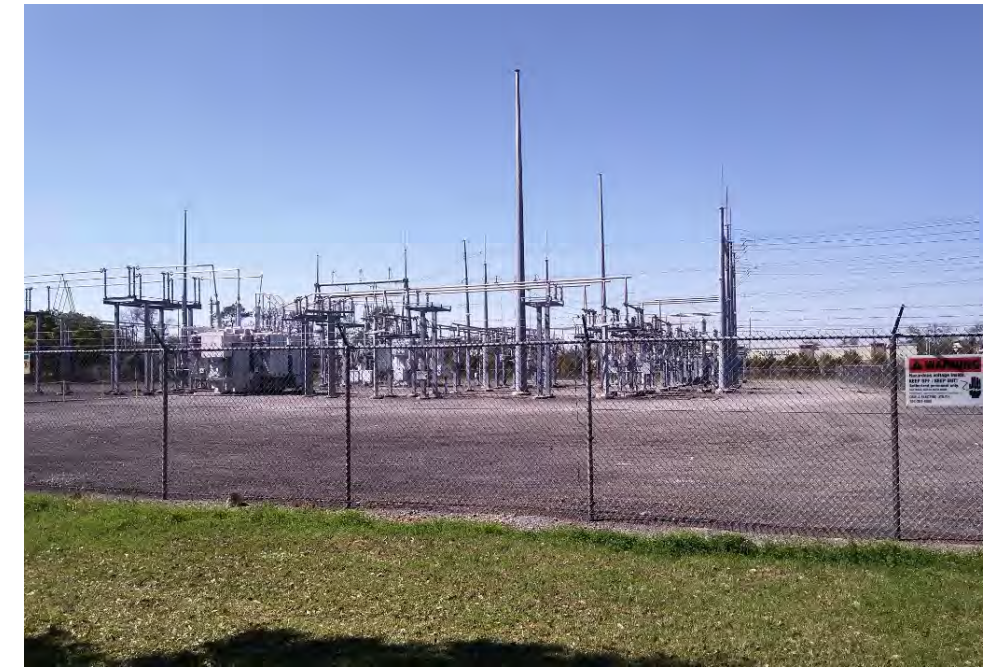
View of the electrical substation facility.
