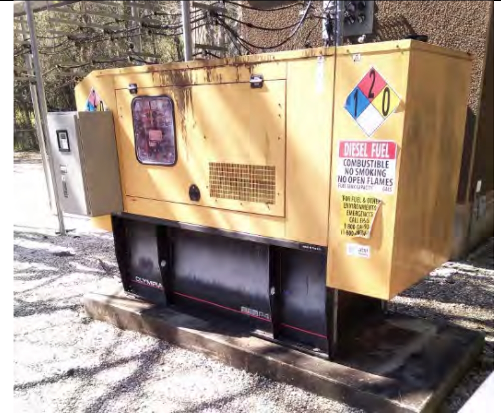
View of first emergency generator tank on-site.
