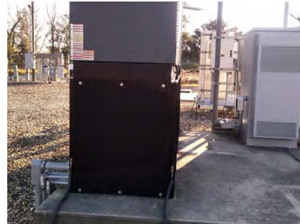
View of an emergency generator diesel tank.
