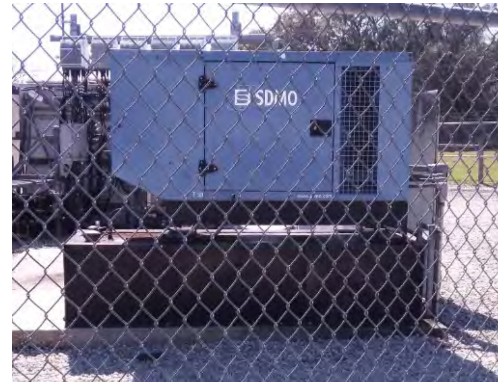
View of second emergency generator diesel tank.
