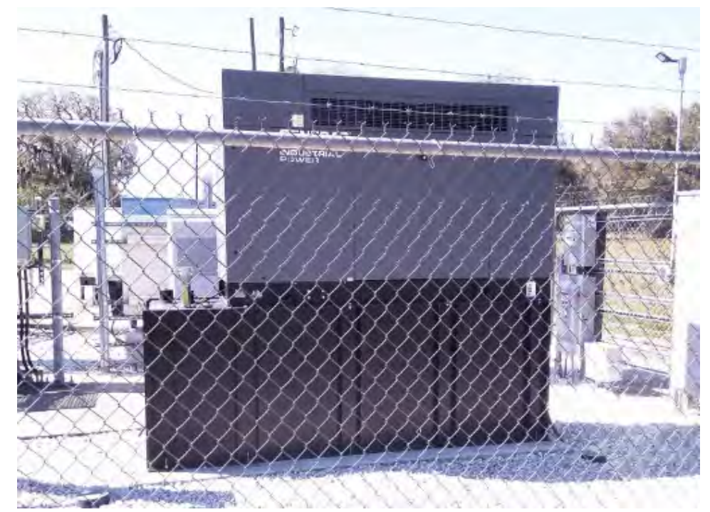
View of first emergency generator diesel tank.
