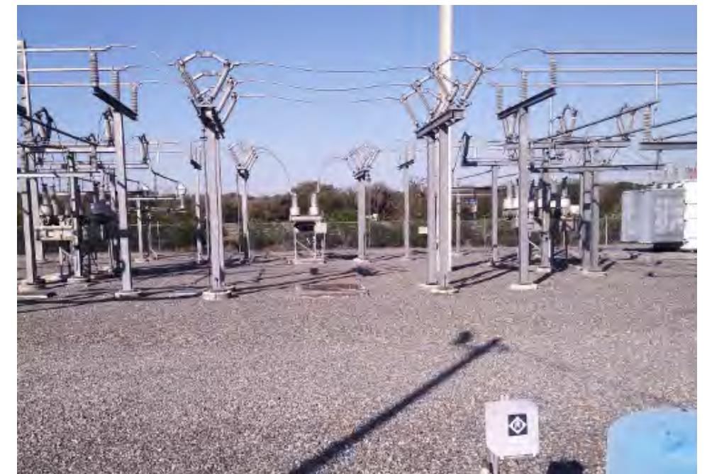
View of the electrical substation.
