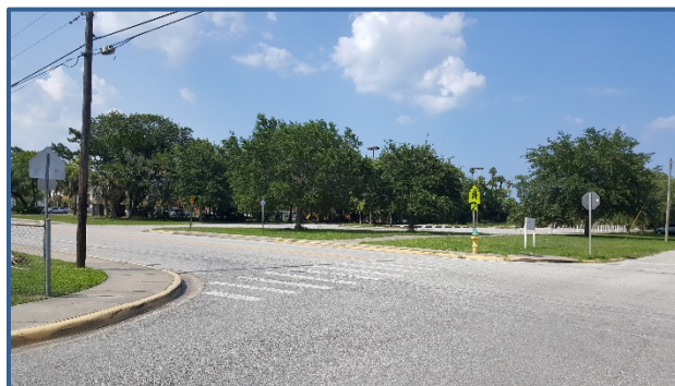
There are no ADA accessible sidewalk ramps at Loomis Ave and Keech St.
