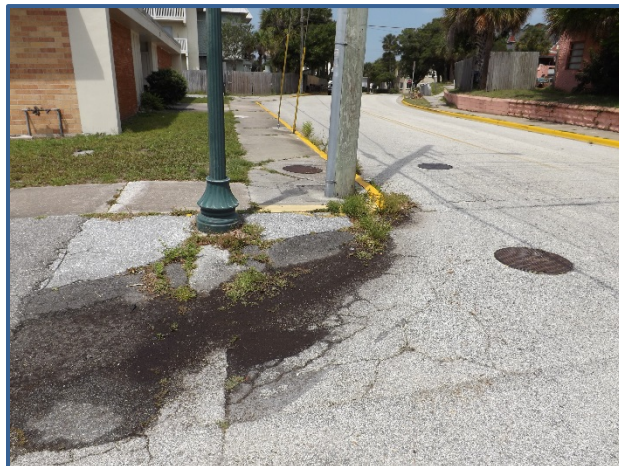
The southwest curb of Hollywood Ave lacks an ADA accessible sidewalk ramp at Harvey Ave.
