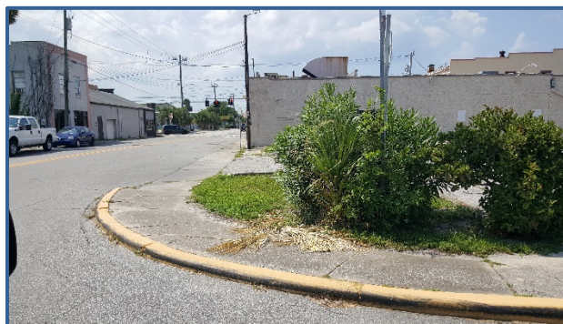
There are no ADA accessible sidewalk ramps at the intersection of Beach St and Michigan St.
