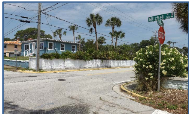
There are no ADA accessible sidewalk ramps at the intersection of Halifax Ave and Mitchell Pl.
