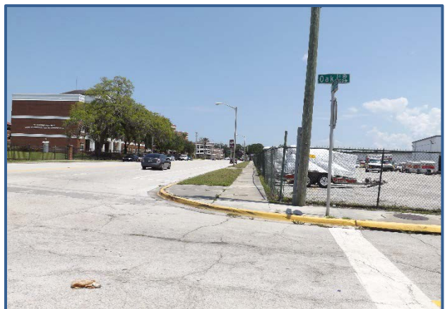
There are no ADA accessible ramps at the intersection of Lincoln St and Oak St.
