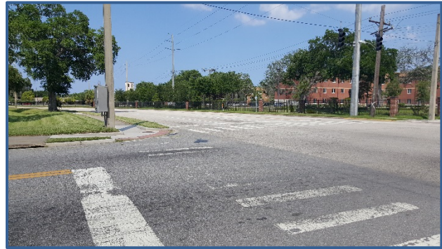
A faded existing marked crosswalk at Dr. MLK, Jr. Blvd.
