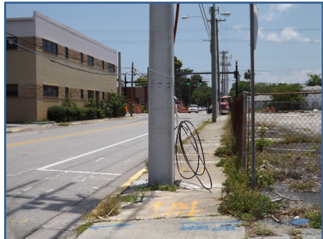
Utility pole infrastructure and wiring obstructing the sidewalk on Seagrave St.
