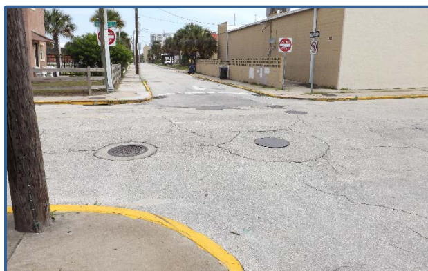
There are no ADA accessible sidewalk ramps at the intersection of Coates St and Harvey Ave.
