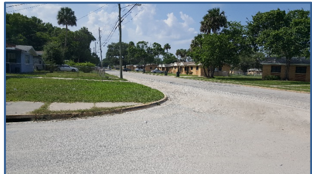
There are no ADA accessible sidewalk ramps at the intersection of Loomis Ave and Caroline St.
