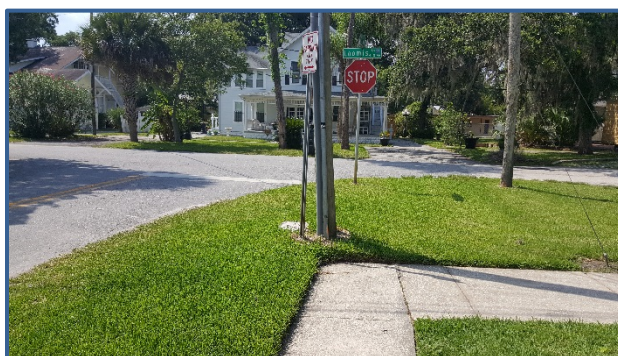
The sidewalk does not extend to the curb at the intersection of Loomis Avenue and Gardiner Court.
