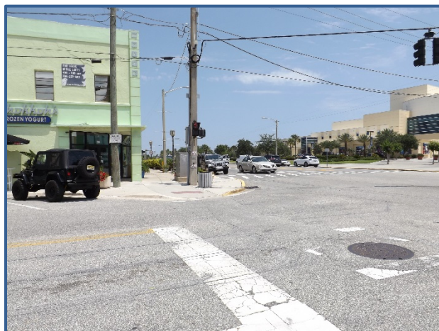
A faded marked crosswalk at Beach and Bay St.
