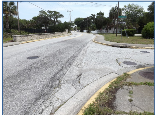
There are no ADA accessible sidewalk ramps at the intersection of Halifax Ave and Harvey Ave.
