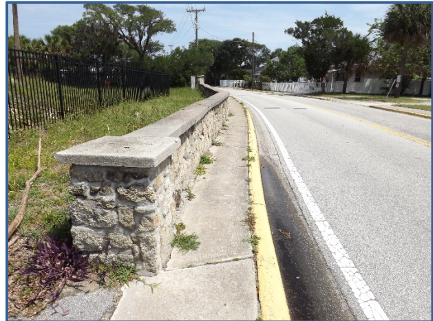
A retaining wall compromises the sidewalk width along Halifax Ave.
