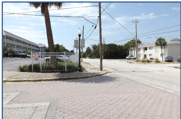
The intersection of Peninsula Dr and Harvey Ave lacks ADA accessible sidewalk ramps.
