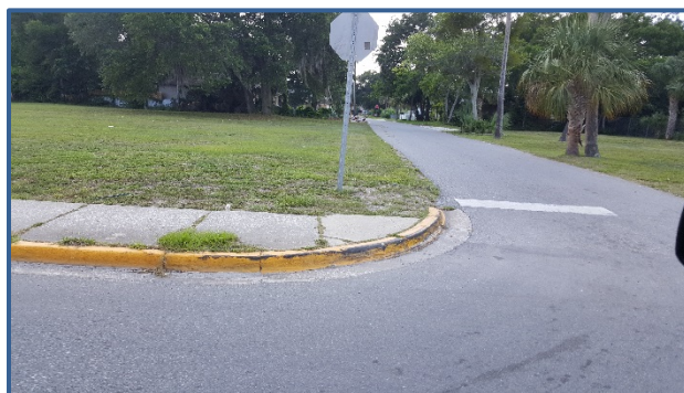
There are no ADA accessible ramps at the intersection of Dr. MLK Blvd and Verdell St.
