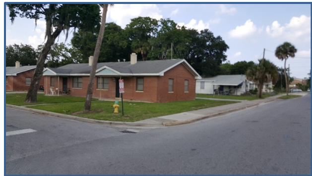
The northeast corner of Loomis Ave and Hudson St is lacking an ADA accessible sidewalk ramp.
