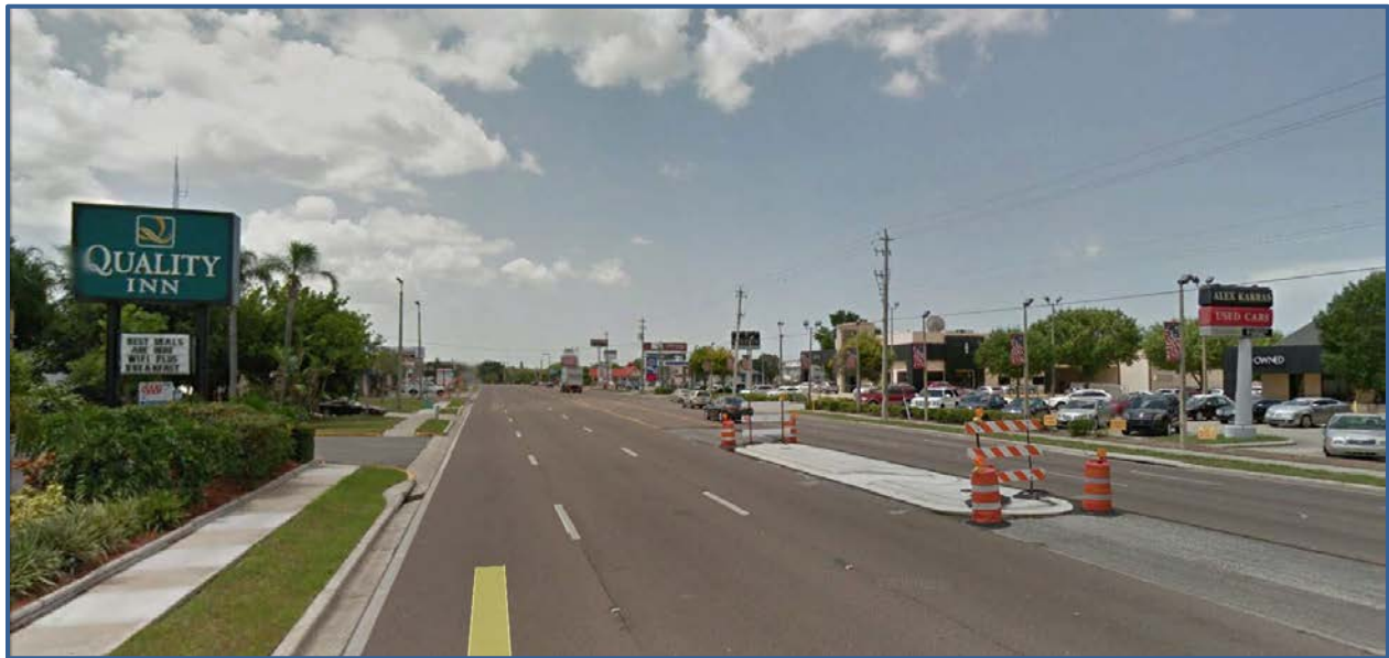
A mid-block crossing under construction on US 41/Tamiami Trail between Florida Blvd and 68th Ave West in Manatee County. Photograph, courtesy of Google Streetview and dated July 2015.
