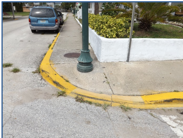
A street light fixture obstructs a sidewalk ramp at Oleander Ave and Harvey Ave.
