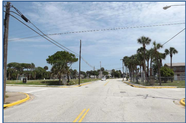
The intersection of Grandview Ave and Braddock Ave lacks ADA accessible sidewalk ramps.
