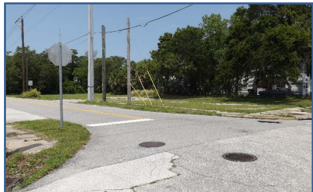
There are no ADA accessible sidewalk ramps at the intersection of Mulally St and Daytona St.
