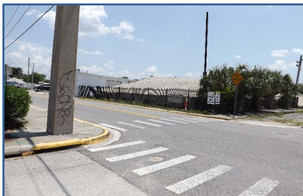
There are no ADA accessible ramps at the intersection of Seagrave St and Mulally St.
