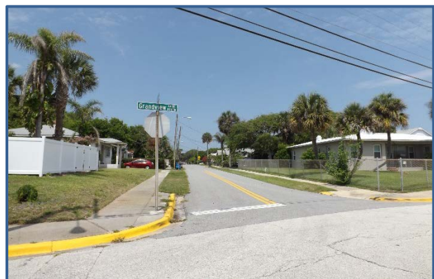
The southwest corner of Grandview Ave and Sears Ave lacks an ADA accessible sidewalk ramps.
