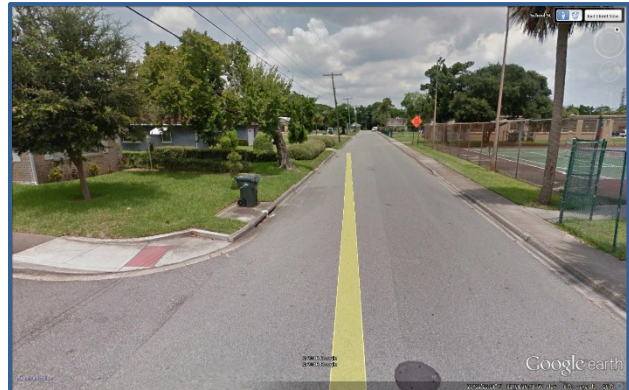
There is no ADA accessible sidewalk ramp on the east side of Henry Butts Dr at Heron St.
