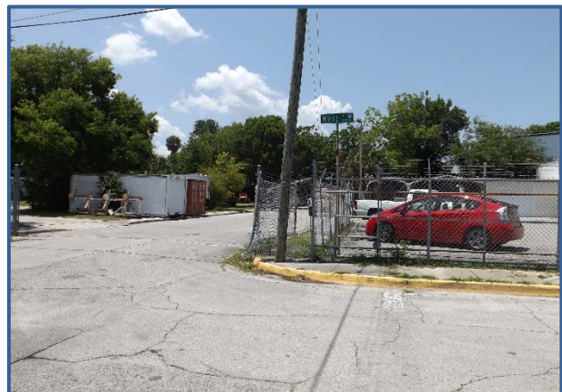
There are no ADA accessible ramps at the intersection of Emmet and West Sts.
