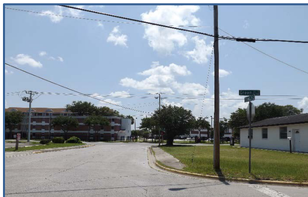
There are no ADA accessible ramps at the intersection of Green St and Third Ave.
