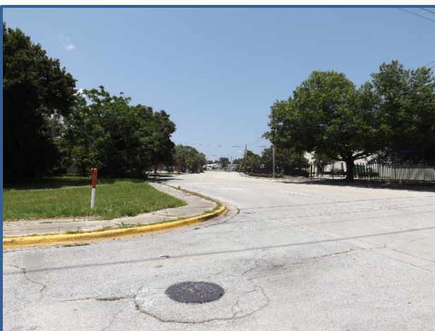
There are no ADA accessible sidewalk ramps at the intersection of Charles St and Weaver St.
