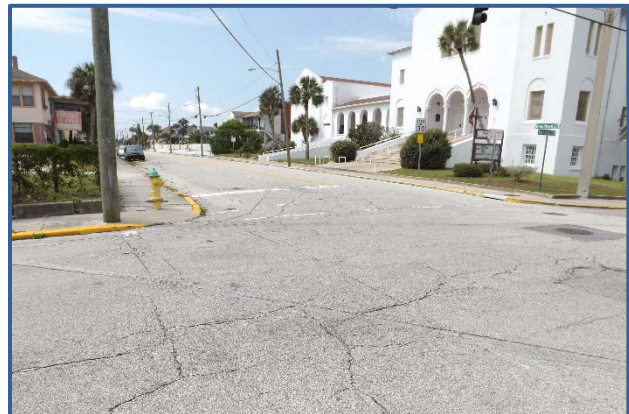
A faded crosswalk at the intersection of Grandview Ave and Harvey Ave.
