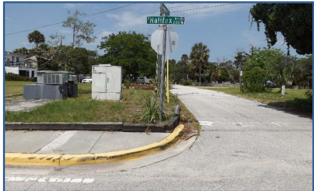
The intersection of Halifax Ave and Hewen Pl lacks ADA accessible sidewalk ramps.
