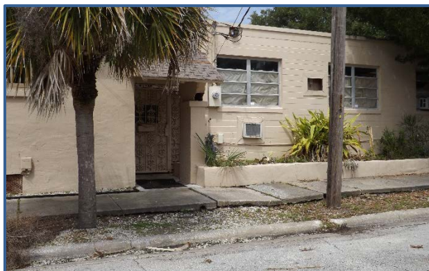
The sidewalk is damaged along Wild Olive Ave.
