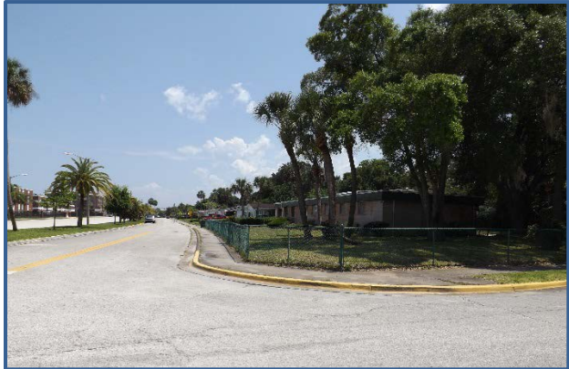
There are no ADA accessible ramps at the intersection of Lincoln St and State St.
