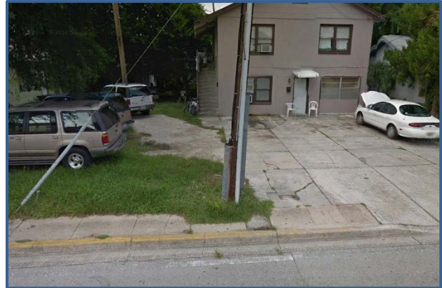
Just east of US 1/Ridgewood Ave, the sidewalk width on the north side of Fairview Ave is not ADA compliant.
