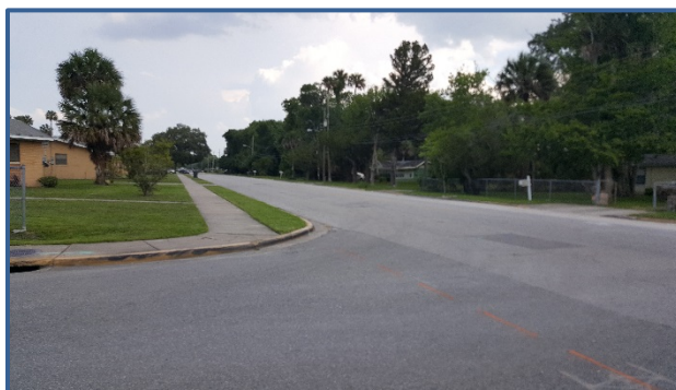
There are no ADA accessible sidewalk ramps at Maley and Caroline Streets.
