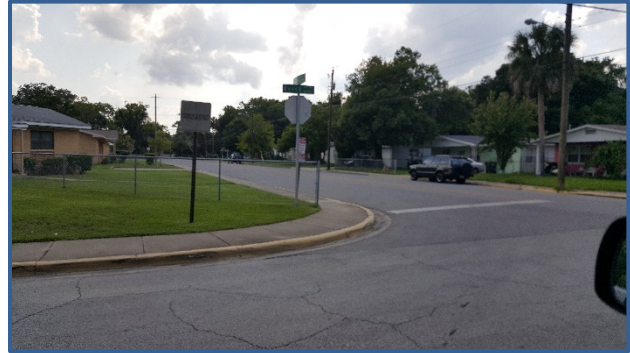
There are no ADA accessible sidewalk ramps at Maley St and Keech St.
