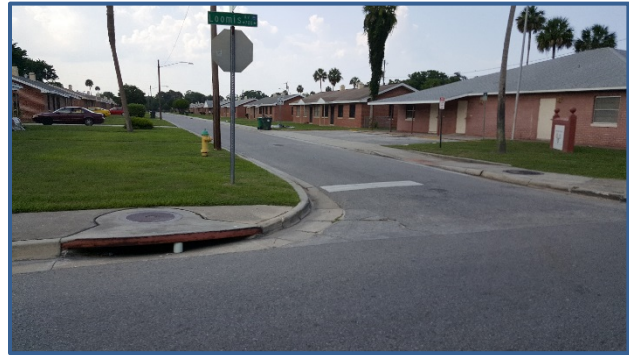
There are no ADA accessible sidewalk ramps at the Loomis Ave and Whitney St intersection.
