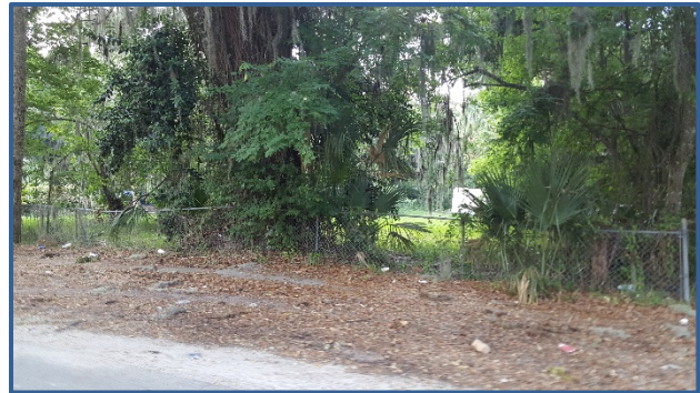
A stretch of broken sidewalk on Maley St.
