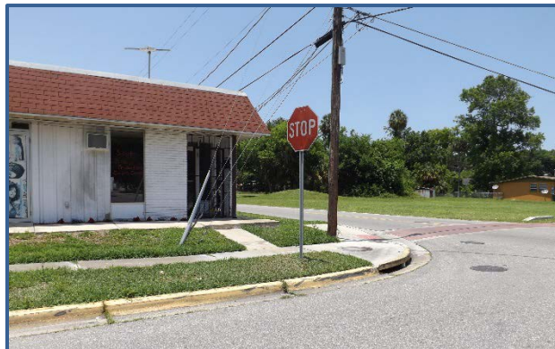
There are no ADA accessible ramps on the west side of the Jean St and Magnolia Ave intersection.
